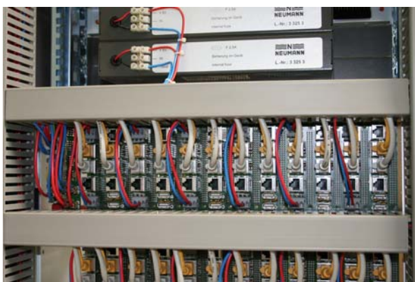
Panel backplanes using patch cables
